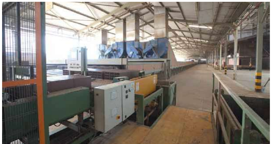
Fig. 1 Cutter placed in the front of two parallel dryers
