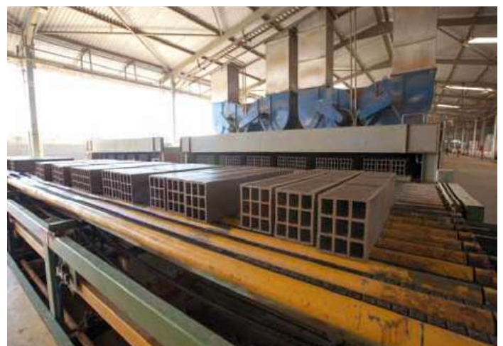
Fig. 3 Exit of two parallel dryers
