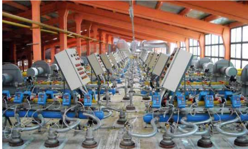
Fig. 1 Gas combustion plant installed on a tunnel kiln
